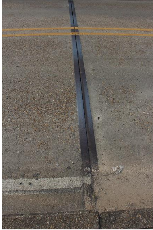
Condition Photo 14: Expansion joint closed at one end and open at the other, bent 5.
