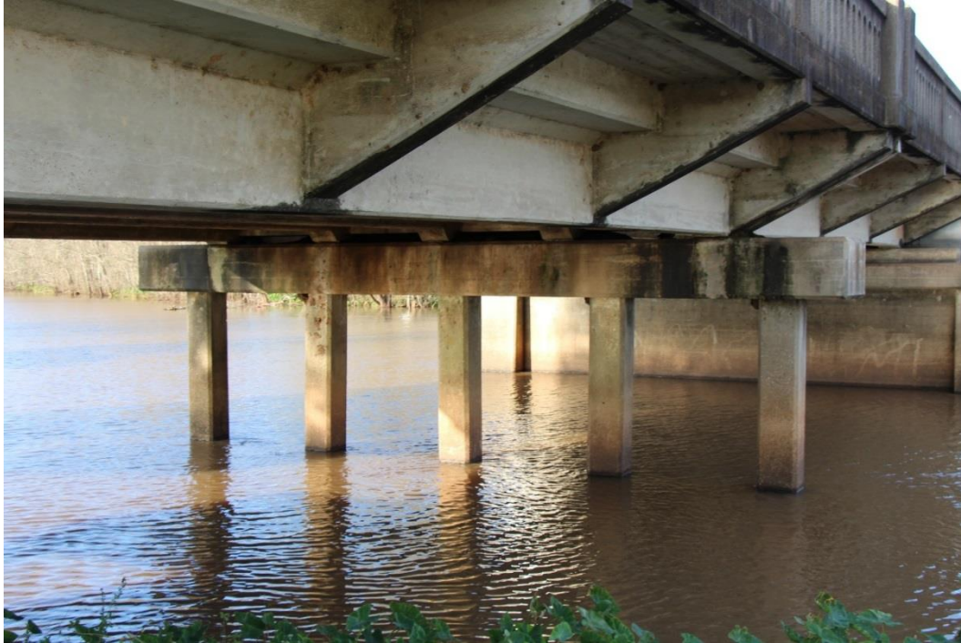
Condition Photo 16: Water staining of concrete bent and piles, bent 3.
