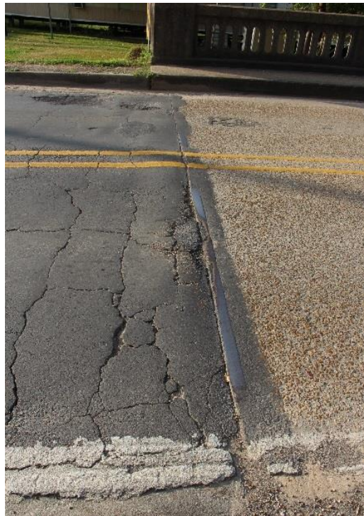
Condition Photo 15: Asphalt joint at south end of bridge.
