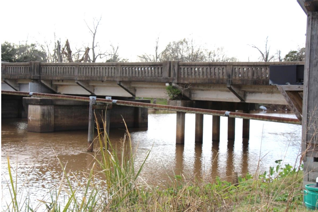
Condition Photo 4: Overview of concrete approach spans, spans 5 and 6, exhibiting watering staining.
