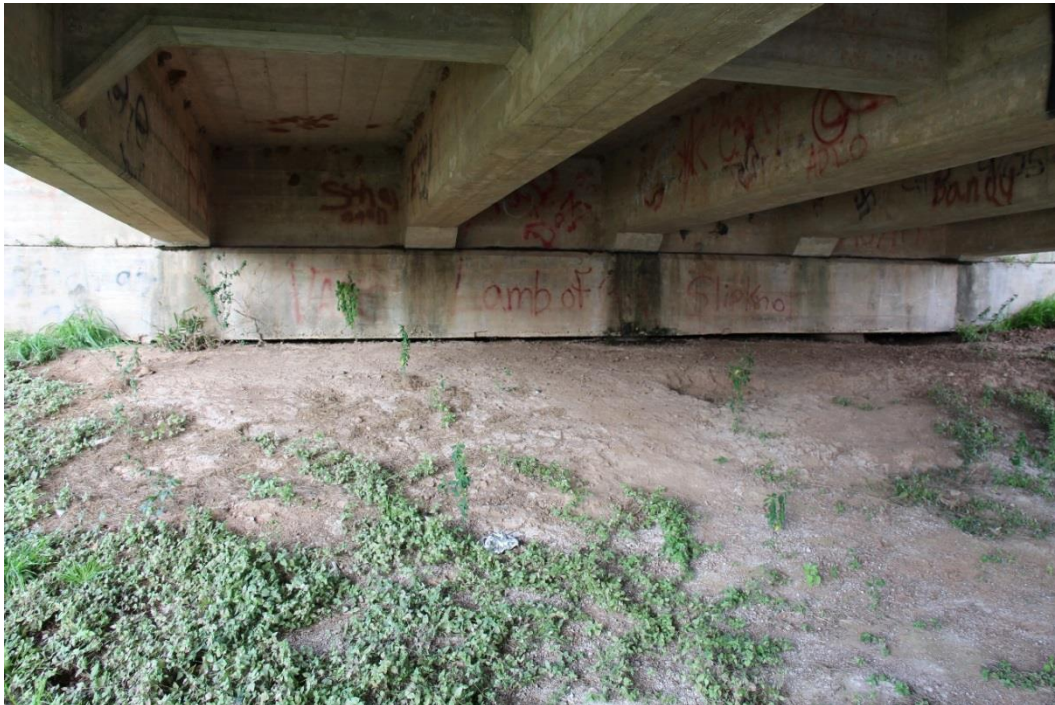
Condition Photo 5: Exposed concrete piles at end bent 1; also showing graffiti.
