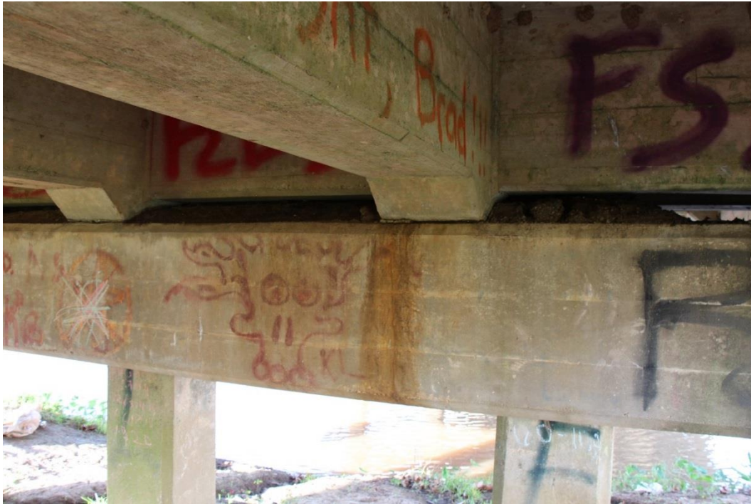
Condition Photo 8: Graffiti on the concrete bent cap, bent 2, piles and beams of the approach span.
