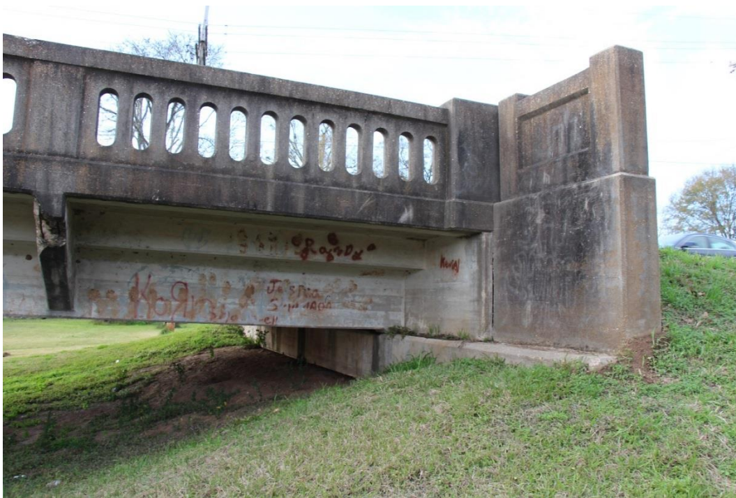
Condition Photo 3: Graffiti on concrete approach span beams, span 7.
