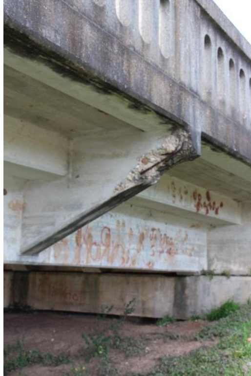
Condition Photo 2: Concrete overhang diaphragm (span 1) spalled with exposed reinforcing.
