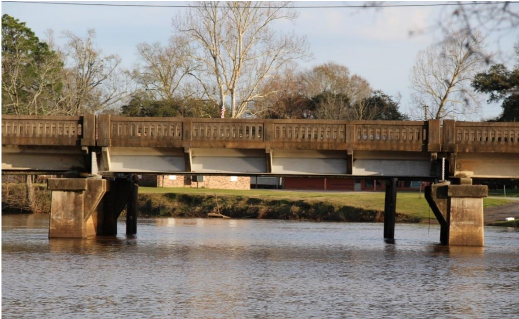
Character-defining Feature Photo 2: Design and construction of the bridge superstructure. The steel I-beam main span was designed to be removable.
