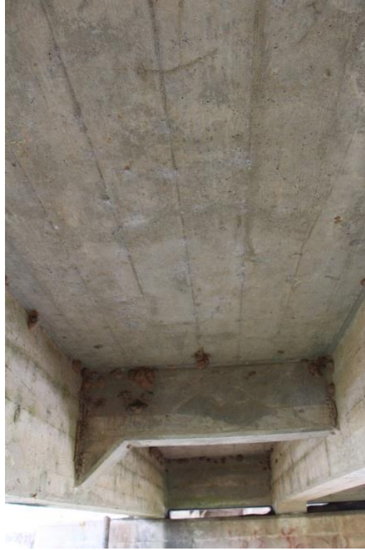
Condition Photo 6: Typical condition of the underside of the concrete deck and concrete deck girders for the approach spans, including several dirt daubers.
